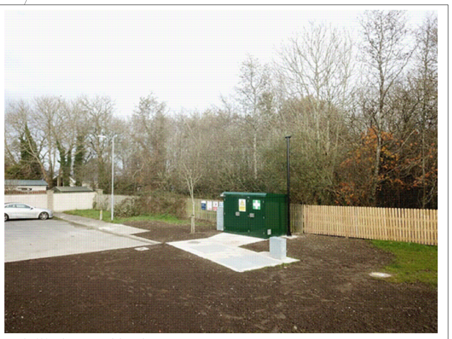
IMAGE 001 - FOUL PUMPING STATION EXAMPLE
